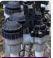
Typical Irrigation Valve
